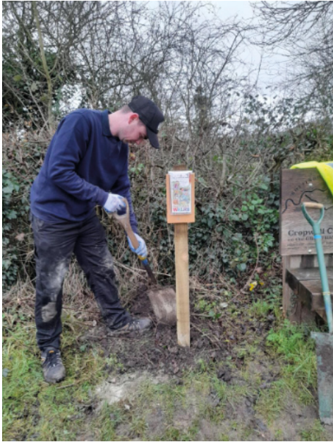
Jake installing one of the two remaining walk leaflet holders at Redmile and Crowwell Bishop.
