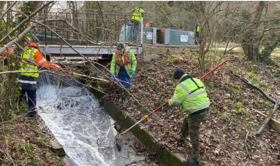
Some photos from a chilly January (clockwise): John T getting down & dirty! Mudlark getting a tow up the canal to carry out some dredging. Volunteers busy working on Denton Weir spillway clearance.
