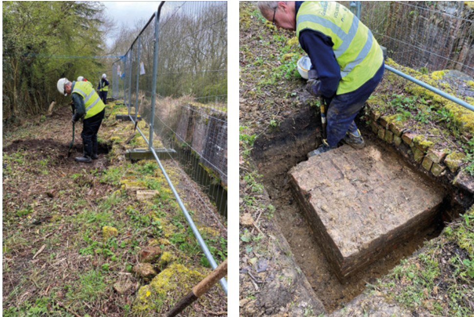
Digging commences at Lock 13 – with exposed buttresses seem to be connected to the lock wall ...
